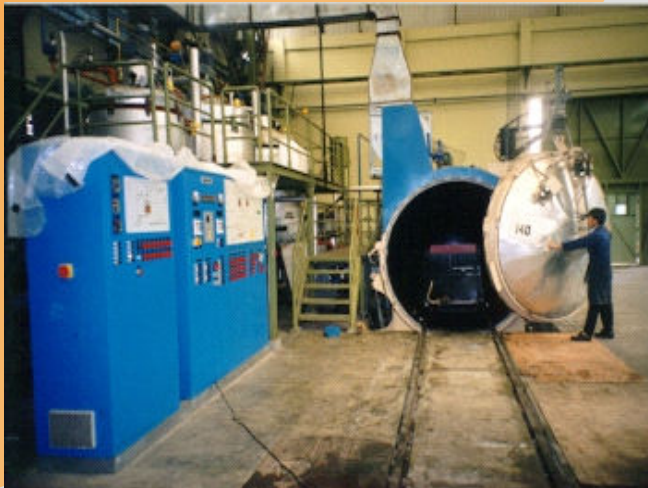
Vacuum Pressure Impregnation
